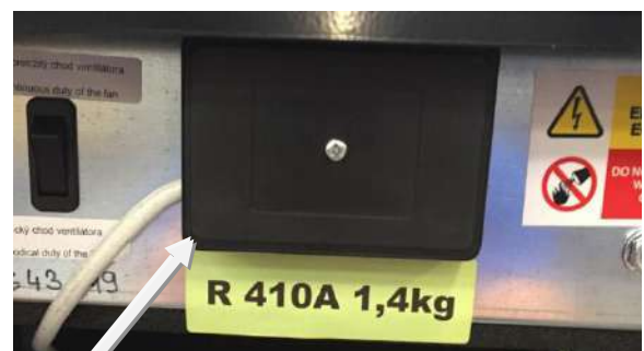
The mains terminal block is located in this black box
